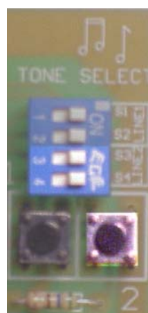
Line 2 switches and test button
